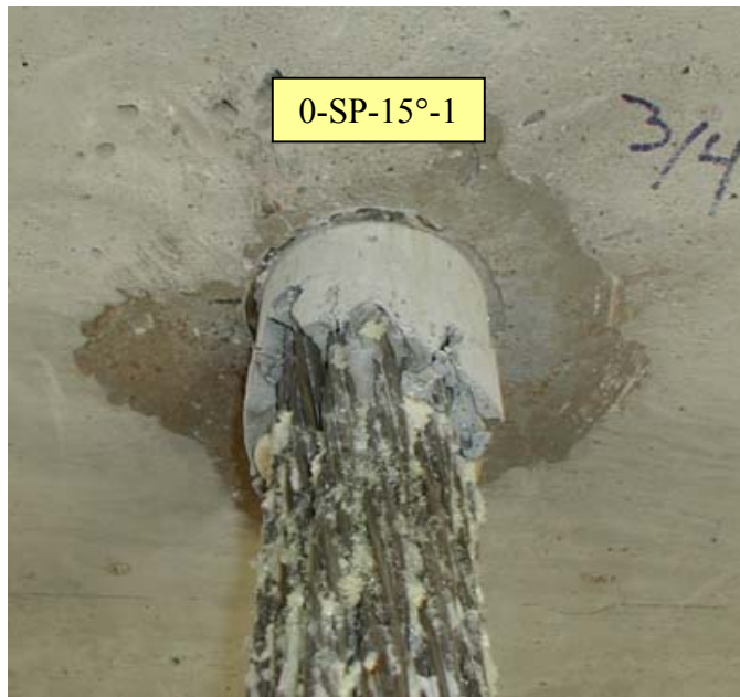
Figure 4-10 Live End of Specimen 0-SP-15°-1 after Testing
